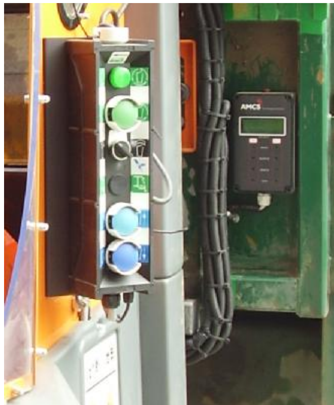
Figure 5 Indicator near operating console
