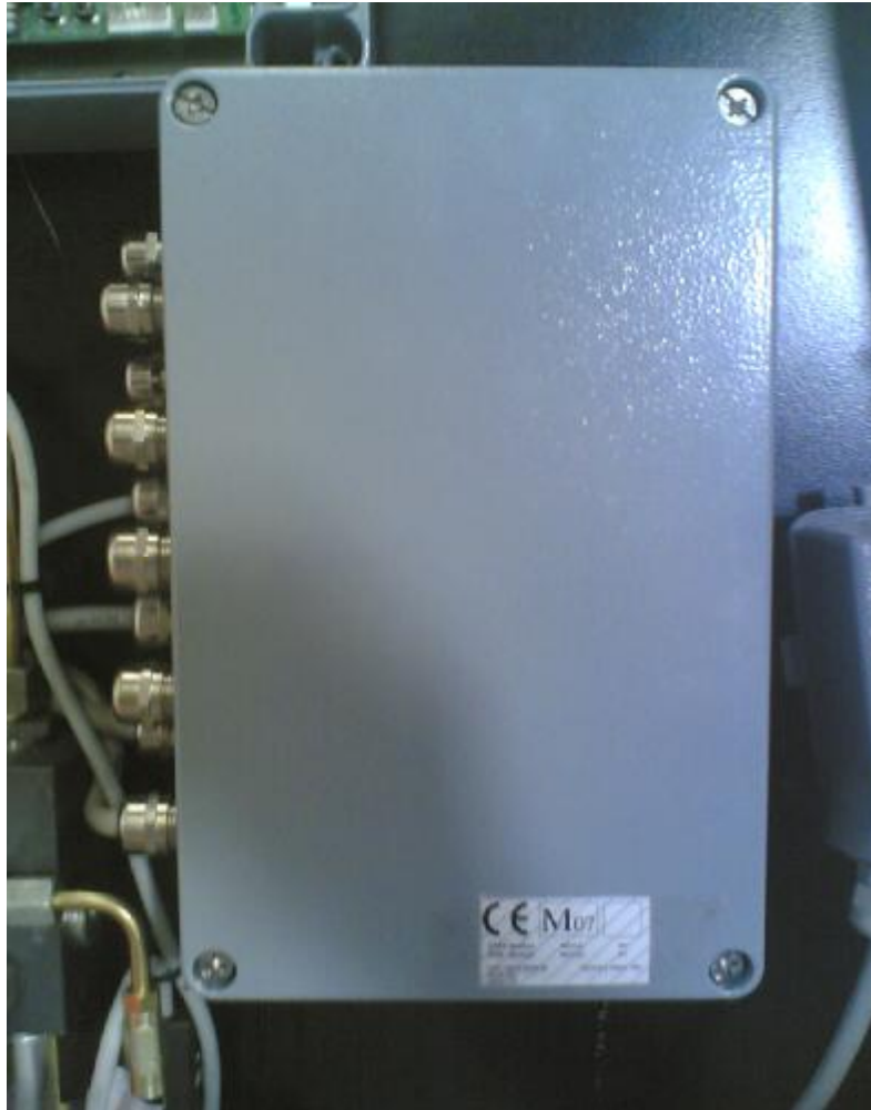
Figure 8 Labelled control enclosure
