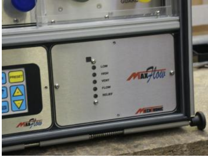
Figure 7 Typical view of special gas extractor control unit (electronic)
