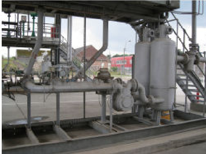
Figure 3 Example of Hydraulics Installation
