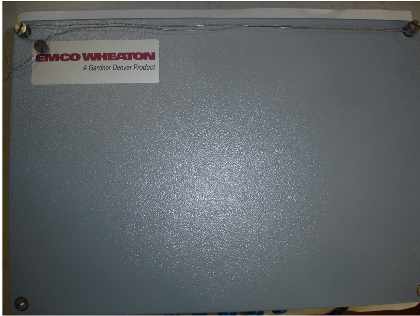
Figure 4 – Sealing of F1031 LC2005 Electronic Register Enclosure
