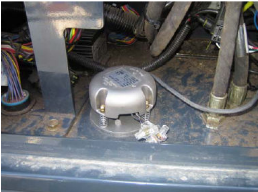
Figure 6 Typical AAA-207109 inclinometer installation
