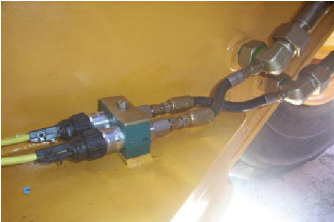
Figure 2 Typical LC965B pressure transducers installation
