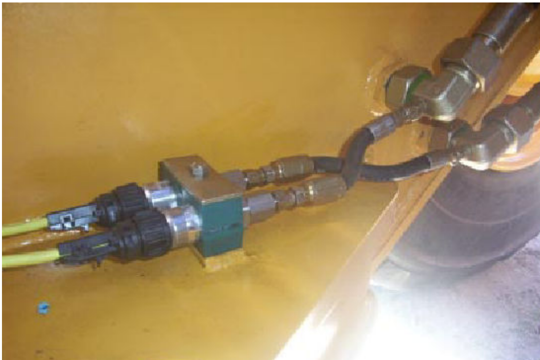
Figure 2 Typical pressure transducers installation
