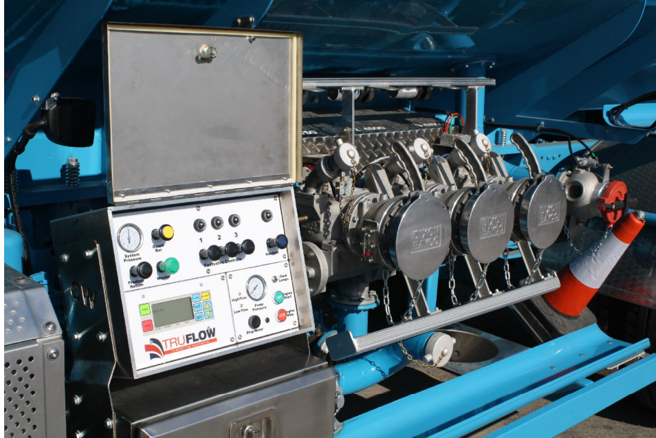
Figure 12 Combined control box
