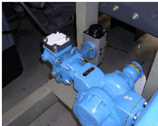
Figure 14 Pneumatic Butterfly Valve
